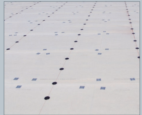
2. Secure a cover board* to the purlins with RetroDriller fasteners and round RhinoBond Plates for membrane attachment. *Additional non-RhinoBond insulation fasteners may be required per FM guidelines, as illustrated by the square plates shown above. Spacing is always specified by the roof system manufacturer.
