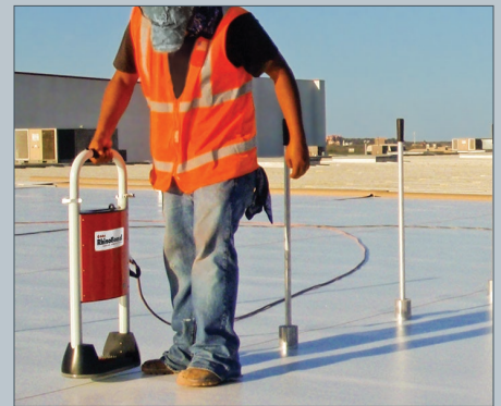
3. After the membrane is installed, weld each plate using the RhinoBond tool.
